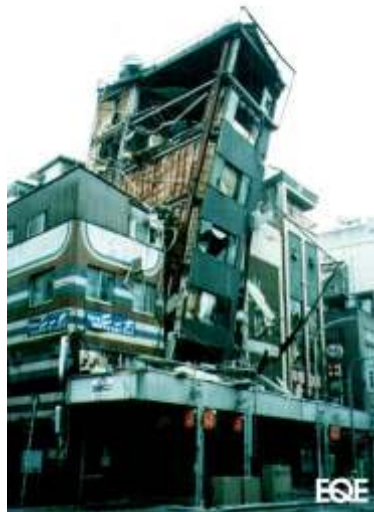
Figure 3: Collapse of a weakly redundant steel building in the slender direction during the 1995 Kobe Earthquake. Picture taken from the web site http://www.eqe.com/publications/kobe/kobe.htm .
