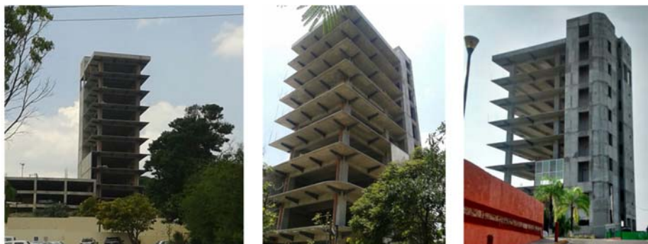
Figure 1: Nine-story building in construction process with only one-bay frame in the slender direction located in Tuxtla Gutiérrez, Chiapas, Mexico.
