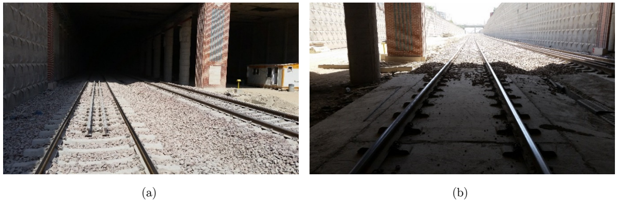
Figure 3: Overview of the test tracks along the transition zone: a) track with auxiliary rails, b) track without auxiliary rails.
