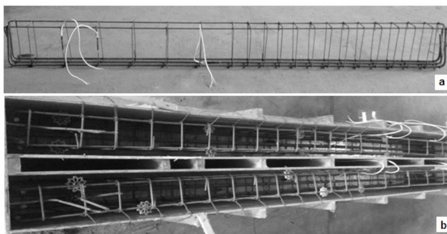
Figure 4: Beams before concrete placement (a - instrumentation of steel bars; b - Molds for beams).
