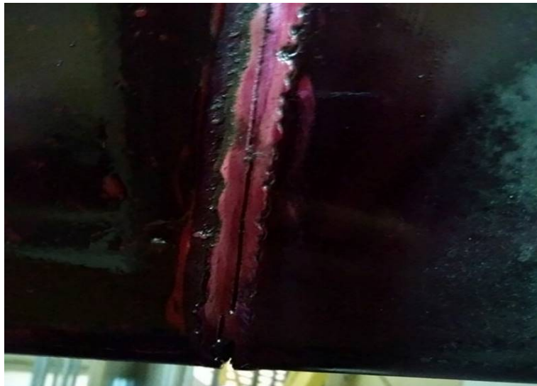
Figure 14: Extended fatigue crack thickness along butt-welded connections.
