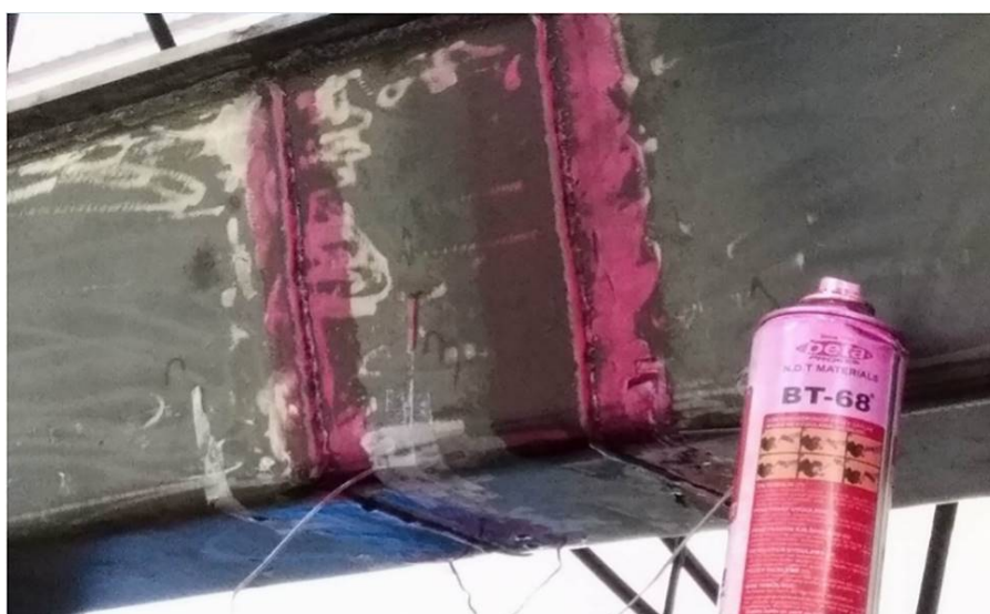
Figure 13: Detection of crack propagation using a dye-penetrant method.
