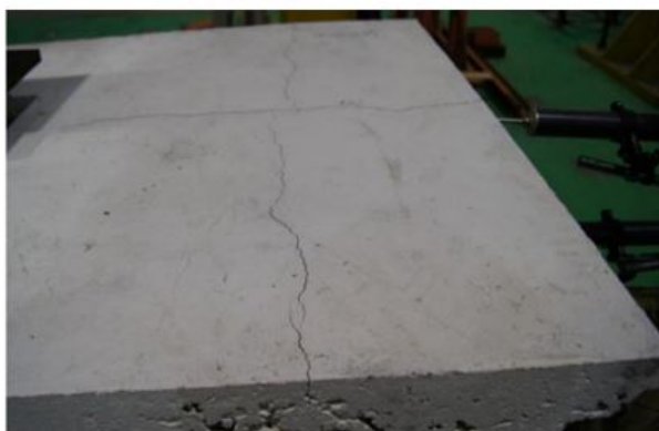
b) Transverse crack at shear span
