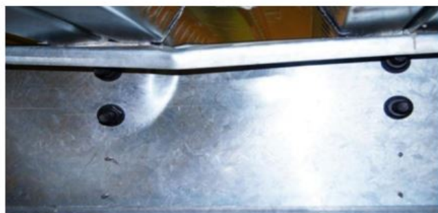
e) Failure of steel beam web
