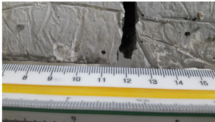
Figure 6. Macro-crack opening measured using graduated scale
