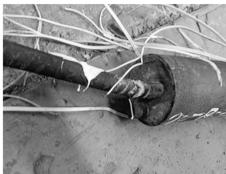
(b) Grout failure of fixed end
