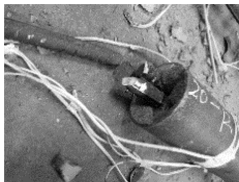
(b) Grout failure of loading end
