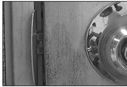
Figure 15 Distortions in the lock.
