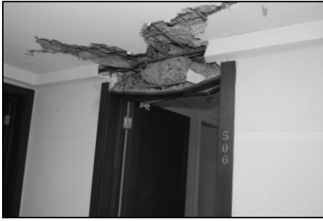
Figure 3 Deflection of lintel above the door
