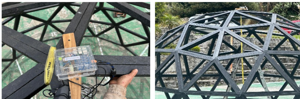
Figure 19 Installation and location of Raspberry Shake 3D.
