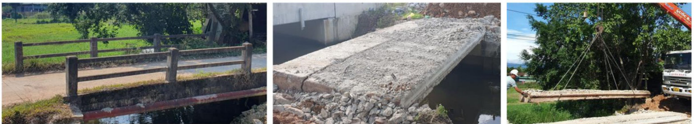
Figure 5 Aged condition of Ben Cho Bridge and retrieval of precast RC slab beams for full-scale experimental testing.
